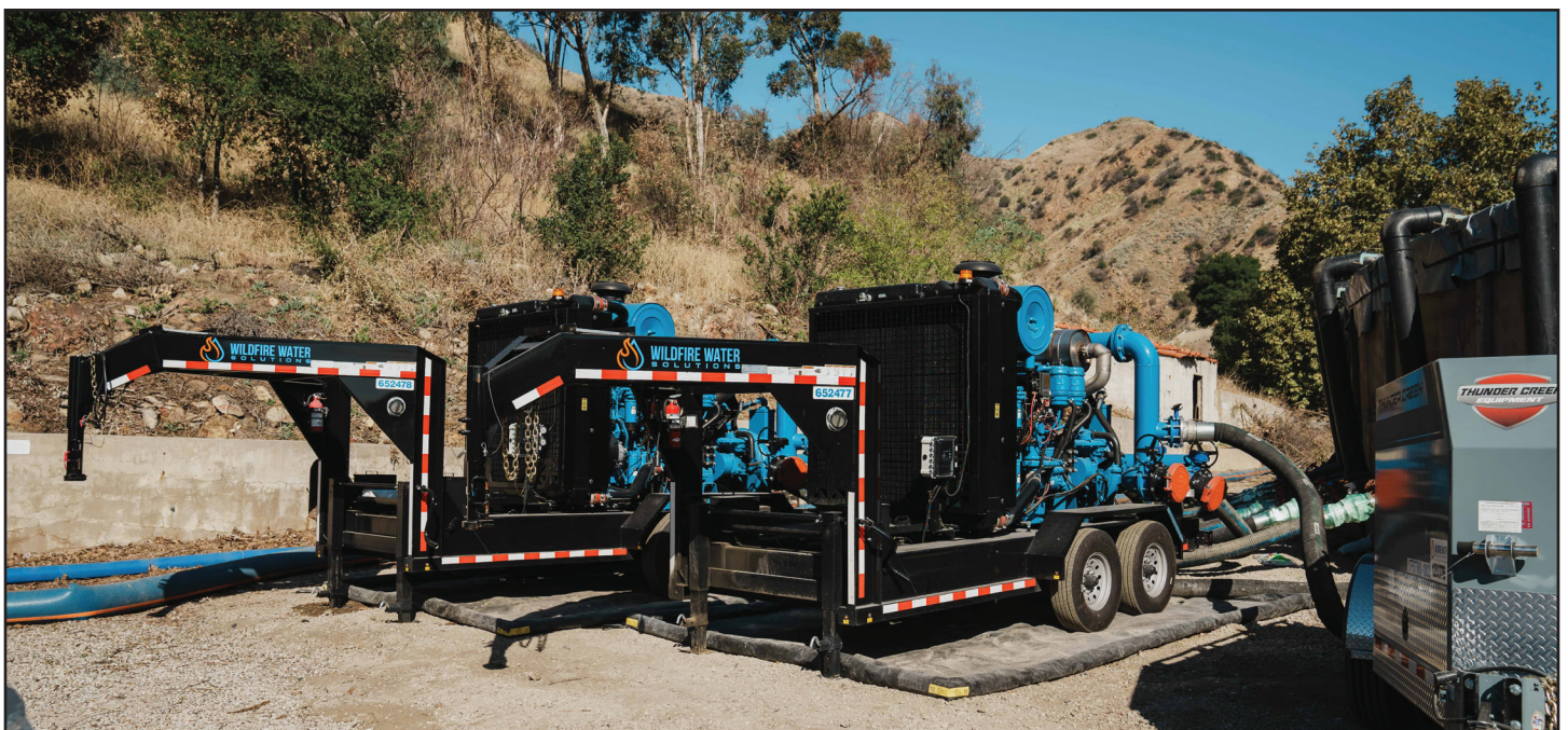
Another view of one of Wildfire Water Solutions' high-capacity diesel pumps.
